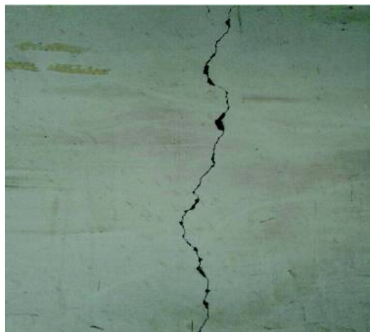
Figure 3: Cracks at juncture of slab and steel beam
