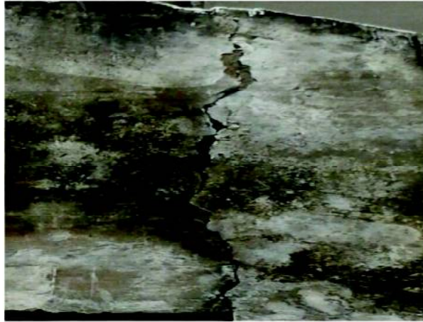
Figure 1: Cracks at juncture of brickwork and steel column
