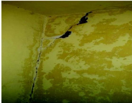
Figure 2: Cracks at corner of sunshade
