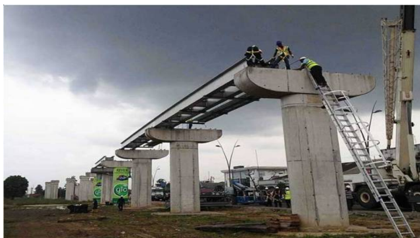
Figure 3: Abandoned monorail project in Port Harcourt, Rivers state
